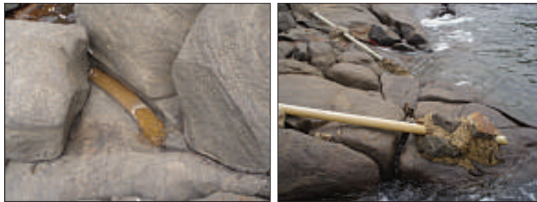
Shit from toilets is discharged on the seashore directly through pipes, which gets in to the seawater during high tides. Sierra Leone
